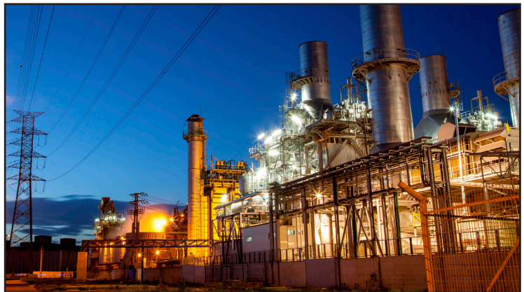
Power Forum: Participants at the 2-day gathering will examine capital project effectiveness in the power industry.
